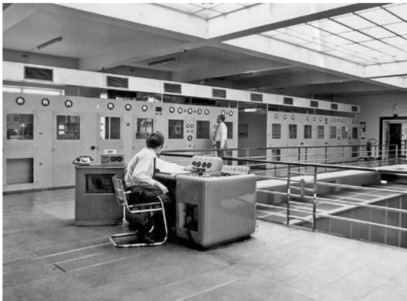
Droitwich 1962: Upper tx hall; replacement longwave tx & control desk
