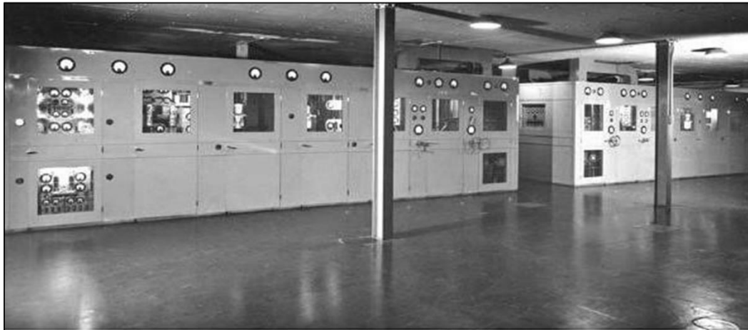
Droitwich 1941: H.P.M.W. (OSE 6) Two 200kw Marconi transmitters operating in parallel.
